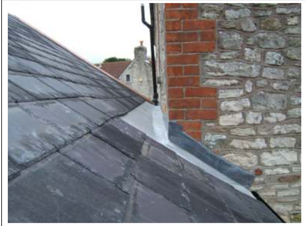
Above: an awkward back gutter abutment
